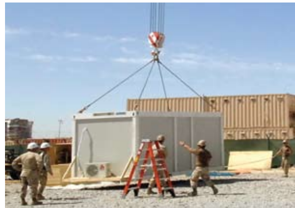
U.S. Navy Seabees direct a crane while moving a relocatable building in Kandahar, Afghanistan
