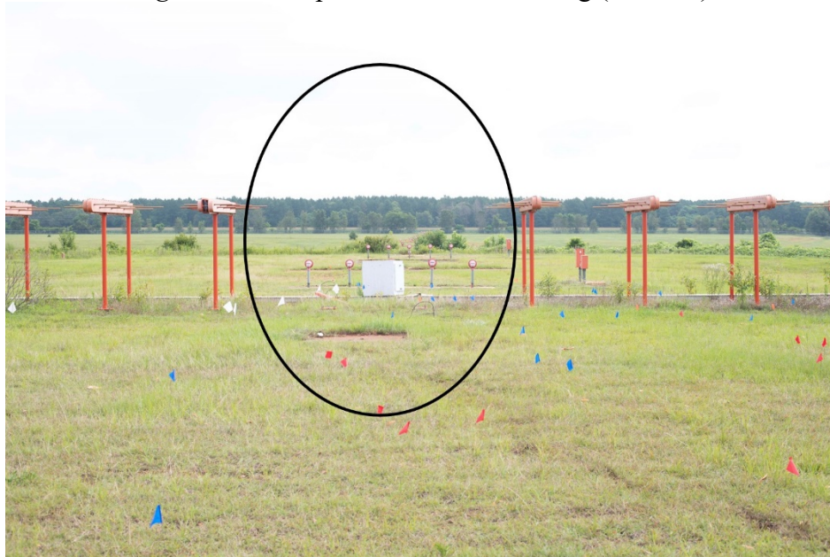
Figure 6: Two missing localizer antennas at the approach end of runway 22R (Tab Z-7)
