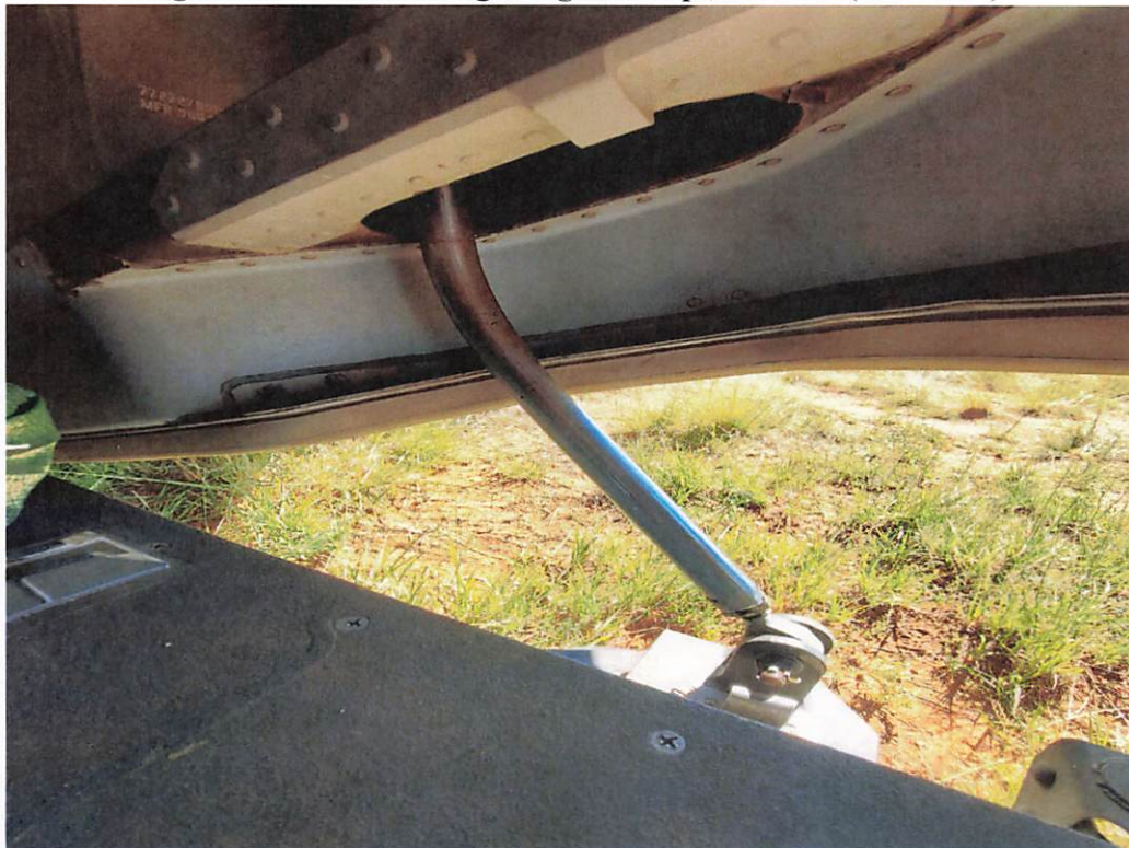
Figure 4-12. MA Damage, Right Ramp Actuator (Tab Z-73)
