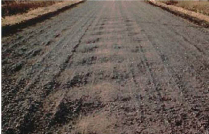
Figure 7-5 (Tab BB-22) Example of Washboarding from US DOT FHA
